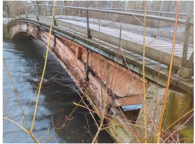
Had to be replaced urgently: the old pedestrian bridge
